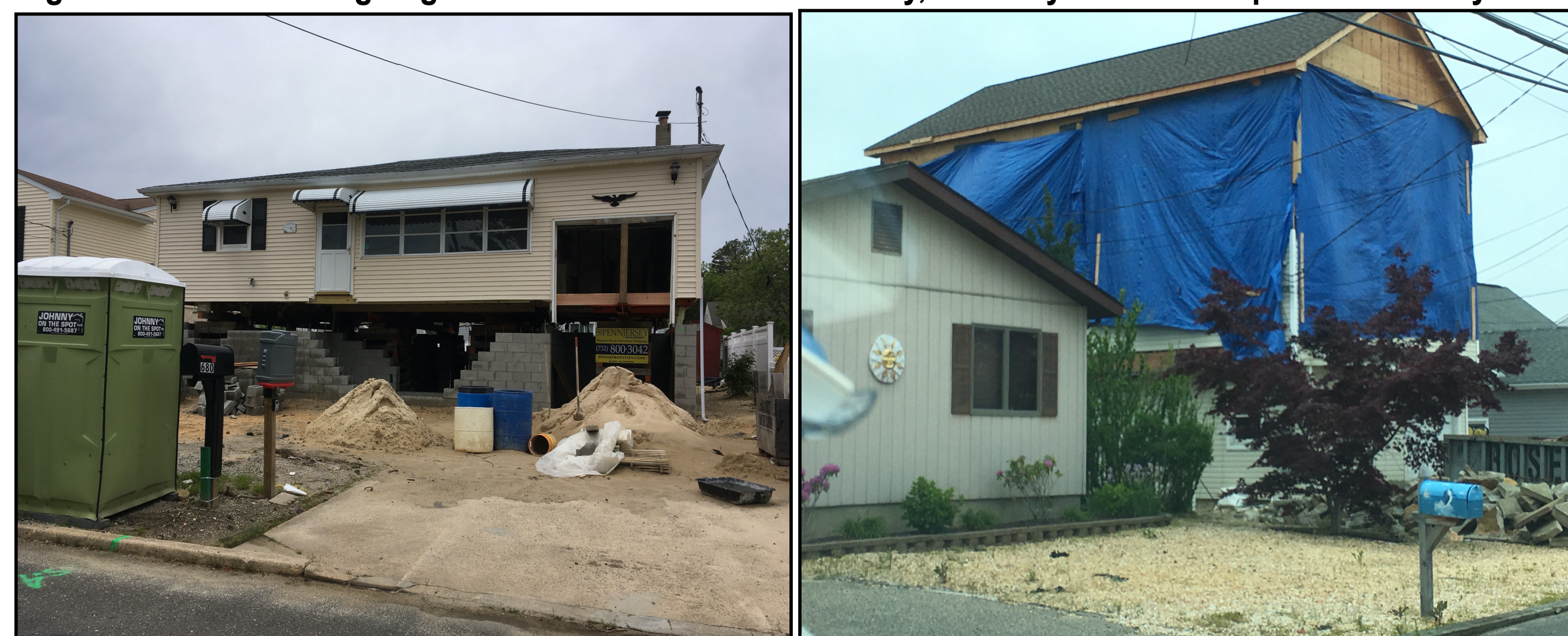
Figure 2. Homes undergoing reconstruction in Ocean County, NJ five years after Superstorm Sandy
